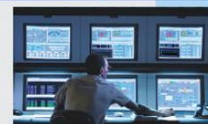
BUILDING MANAGEMENT SYSTEM (BMS) 10
